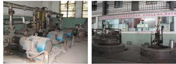
Figure 12 Pumping Motors and Heating Ovens
